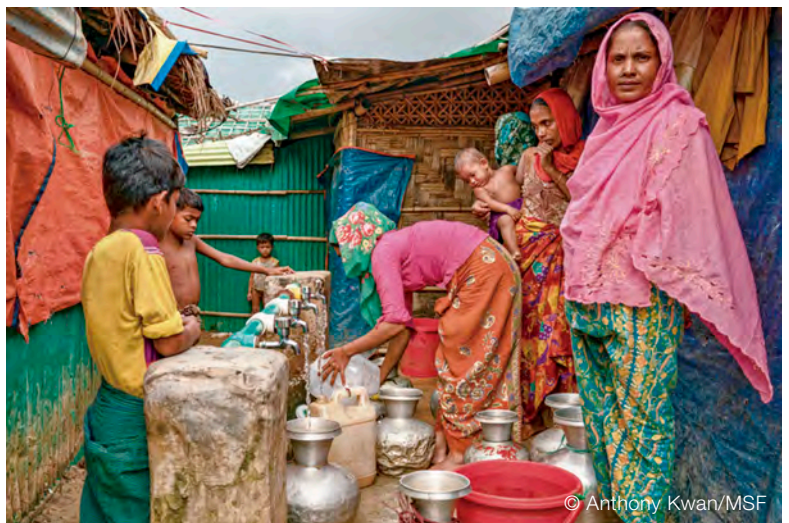
MSF built water and sanitation facilities in Jamtoli camp for Rohingya refugees, Cox's Bazar, Bangladesh.
